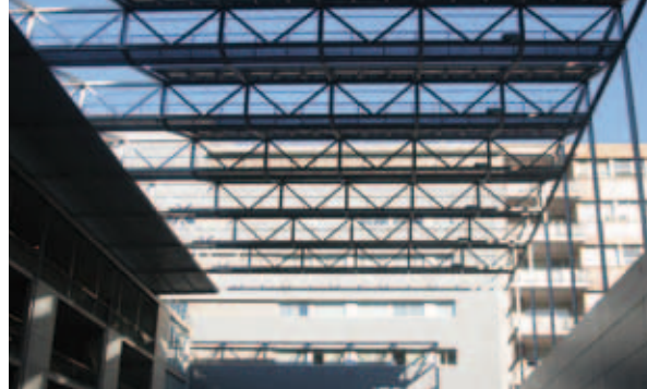
Solar panels of the Faculties of Physics and of Chemistry
