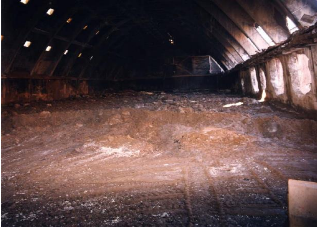
518 519 Figure 10. The silo after the accident. 520
