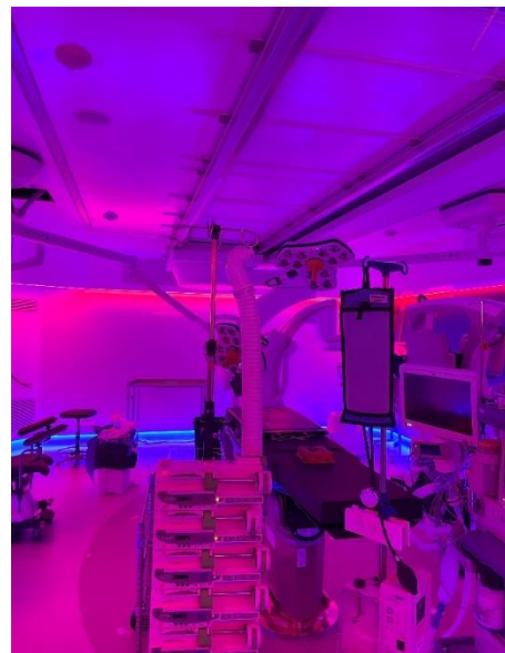
Figure 11 Studied Operating Room from Hospital Clínic de Barcelona
