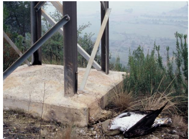
Intensive underline searches allow Bonelli's eagles electrocuted under distribution pylons to be found. Author: CBG-UB).
