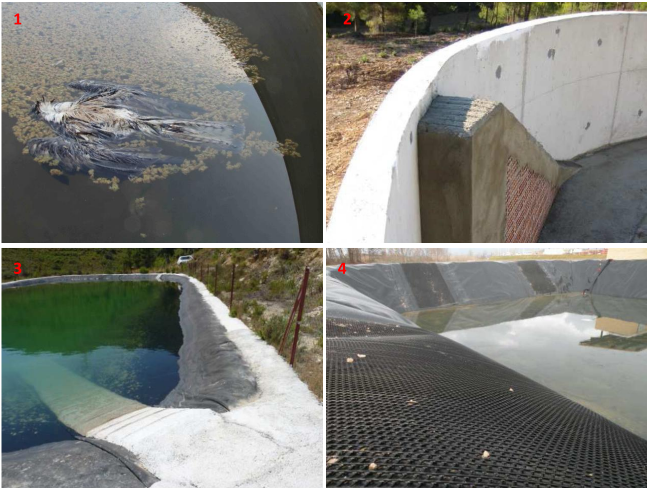
Figure 25: (1) Adult Bonelli's eagle found drowned in a fire prevention water tank; Photo: Francesc Parés (CBG-UB); (2, 3 & 4) Some corrections implemented in Catalonia to avoid wildlife drowning. However, the effectiveness of these corrections, as well as other alternatives, still need to be tested on a long-term basis; Photos: Servei de Biodiversitat i Protecció dels Animals. Generalitat de Catalunya.
