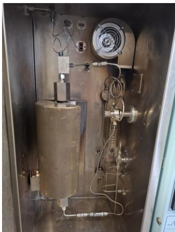
Figure 5: Interior of the Microactivity Reference PID Eng&Tech
