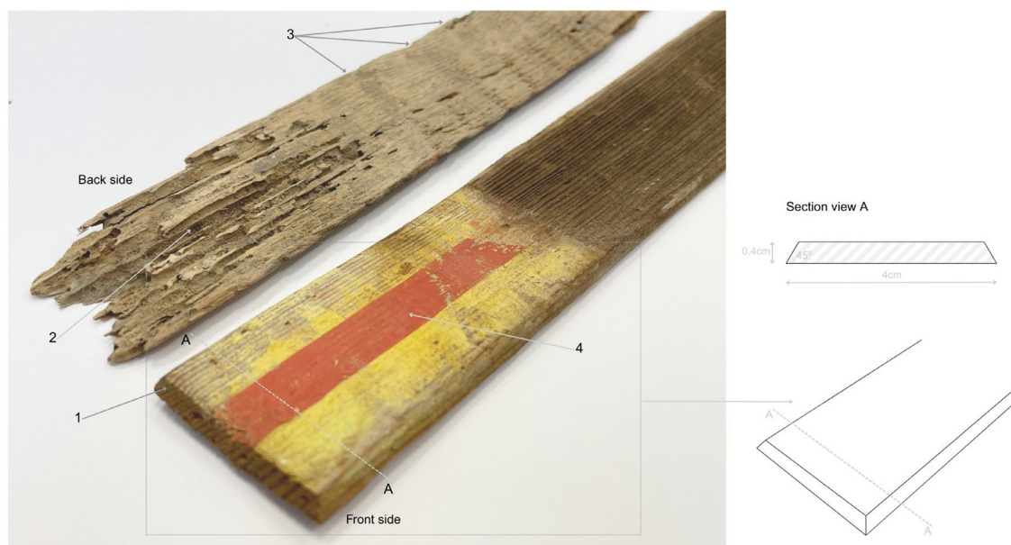
Fig. 2. Front and back side of two joint covers from the ceiling of the Monastery of Pedralbes with evident signs of biodeterioration. (1) Growth rings showing a tangential cut; (2) Tunnels caused by xylophagous insects, resulting in loss of material and density in the wood; (3) Parallel marks from the saw used to cut the strip with which the joint cover was made; (4) Front side with polychromy remains. Faced with a cleaning treatment, the wood of the back side is now as weak and delicate as paper or cardboard.
