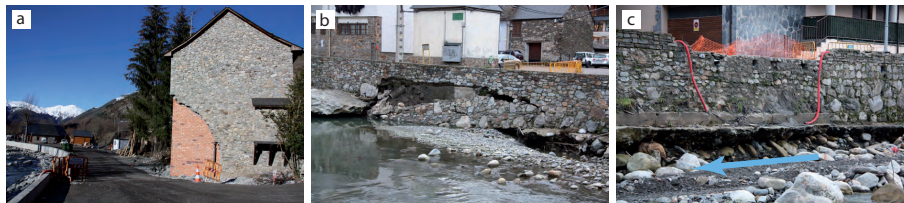
Figure 7. Effects of the 2013 flood event along the Garona River (photos Glòria Furdada, January 2014). (a) A damaged building at Arties by bank erosion that had to be reconstructed. (b) Collapse of a channelization dyke at Les due to vertical incision. (c) Vertical incision in a channelization at Les (the blue arrow indicates flow direction); imbricated clasts below the scoured dyke prove that the Garona River entrenched into its channel bed.
