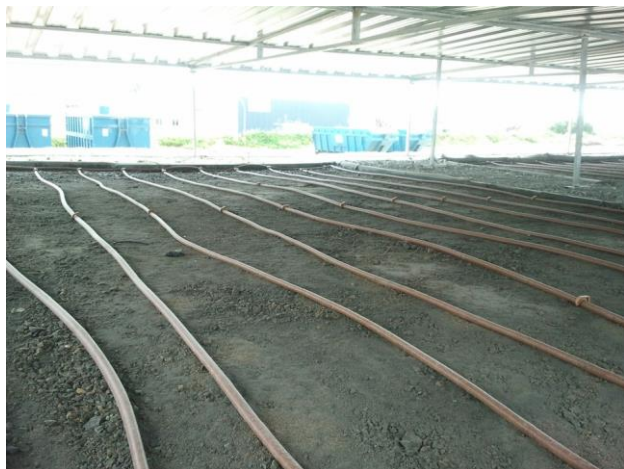
Fig. 2 Set of hoses forming the leaching collection system (LCS) of the three-roads pilot site
