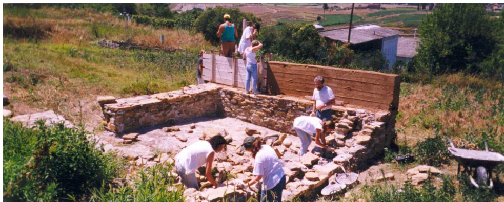
Fig. 12. Building the experimental granary at l'Esquerda in 1998, with P.J. Reynolds standing near the adobe wall
