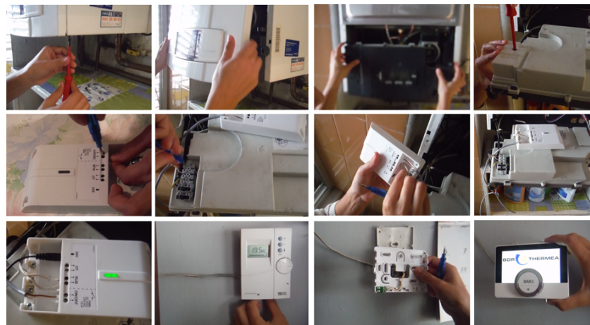
Figure 4. Pictures of the installation of the smart thermostat (BAXI CONNECT) in one of the case study households. The top row shows the removal of the front cover of the boiler. The middle row shows the connection with the gateway. The bottom row shows the new smart thermostat installation.
