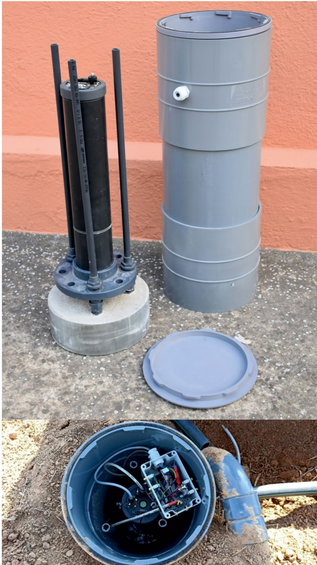
Figure 4. Top: Lemi 44 magnetometer (left) and its bespoke PVC water-proof container (right), which, for the proper leveling and orientation, includes a concrete base to provide stability with leveling foot screws attached with PVC cylinders accessible from the top. Bottom: The magnetometer placed inside its container is buried to attenuate the thermal oscillation. The electronic box on the top contains the data transmission module.
