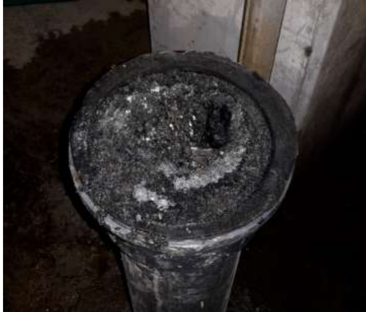
Figure 5.3. Decanter centrifuge drain pipe completely clogged by struvite crystals in Pineda WWTP.
