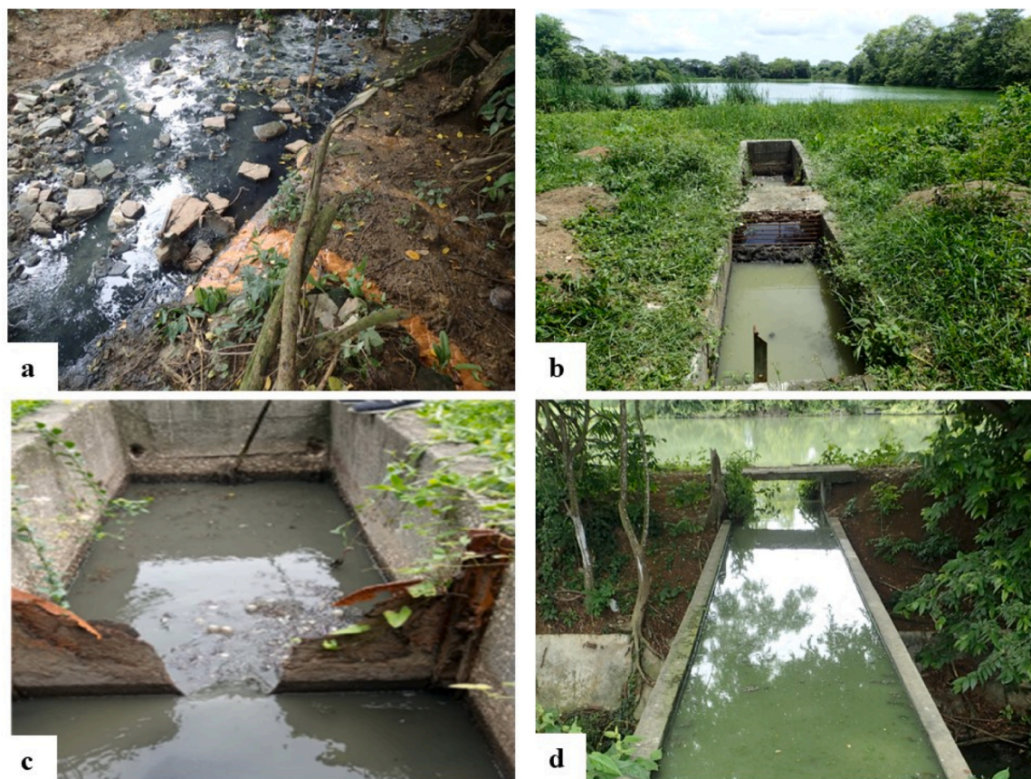
Fig. 3. Pictures of the wastewater treatment system (WTS) of San Antero municipality. A: Wastewater discharge from the WTS into the Cardales stream due to overflow. B: Inlet channel obstructed at the retention grid for solids. C: Wastewater inlet channel showing the concrete weir with hydraulic jump, where the inlet flow was measured. D: Concrete weir between ponds 2 and 3, below which is the outlet channel for the treated wastewater. See location of pictures in Fig. 2. Photographs courtesy of INVEMAR.
