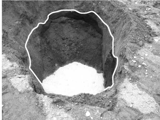
Figure 6 Excavation in a bed clogged for misconstruction of the drainage outlet. The white line stresses the limit between the “clean” sand and the black anaerobic layer. The water of the saturated layer has invaded the bottom of the hole
